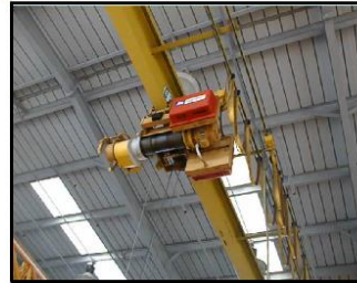
Trolley Mounted Overhead Hoist
